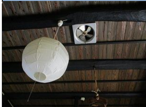
居間天井換気扇
